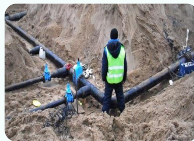
Supply of drinking water
